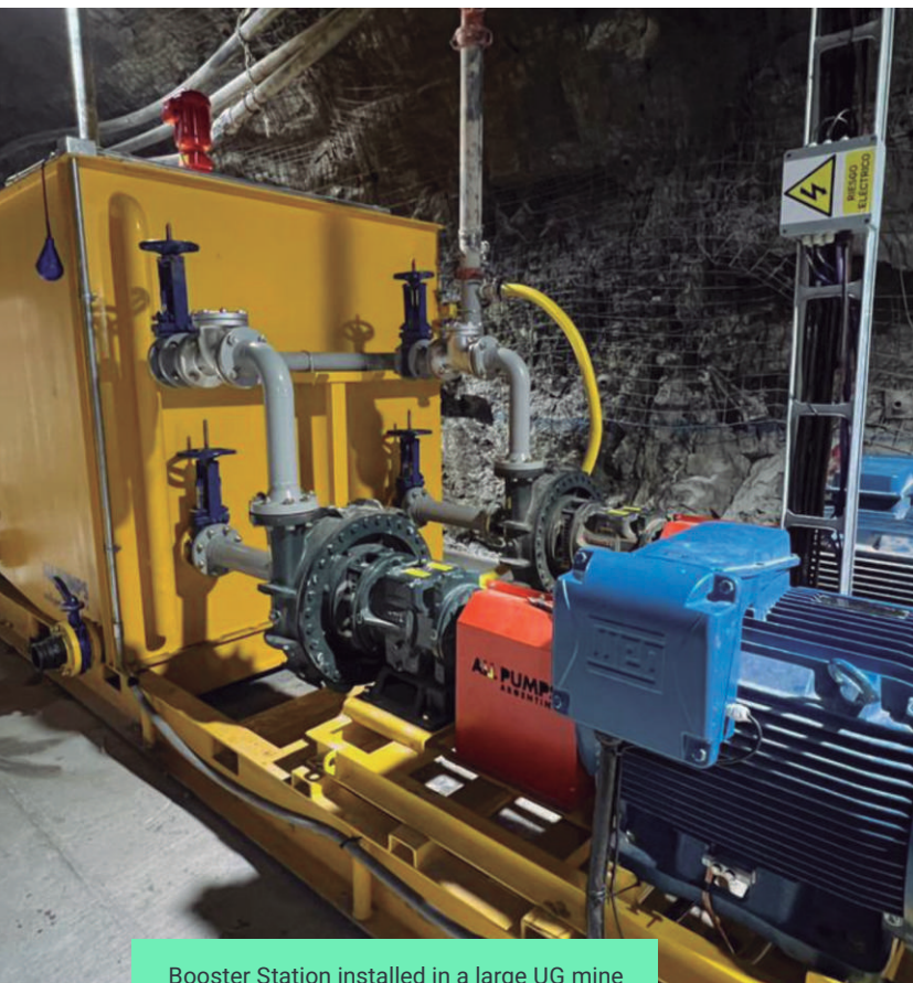
Booster Station installed in a large UG mine located in Santa Cruz, Argentina
